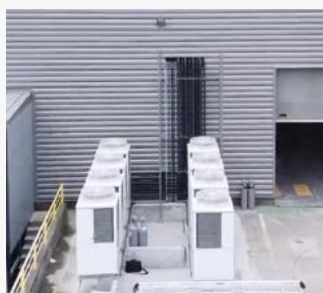
Stemcell Technologies. Global biotechnology company. Saint-Egrève, France. Refrigeration.
