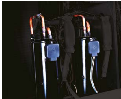
Multiple large-capacity all Inverter compressors (from 14 HP).
